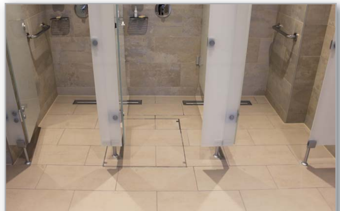
Two Drain+ Compact units draining and supplying three cubicles
