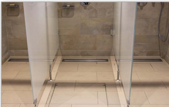
Three Drain+ Compact units installed in cubicle spaces
