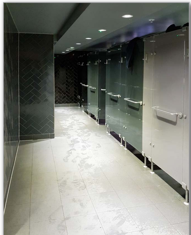
Gymbox changing room and shower facilities
