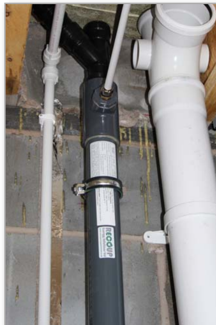
Waste from shower and pre-heat connected
